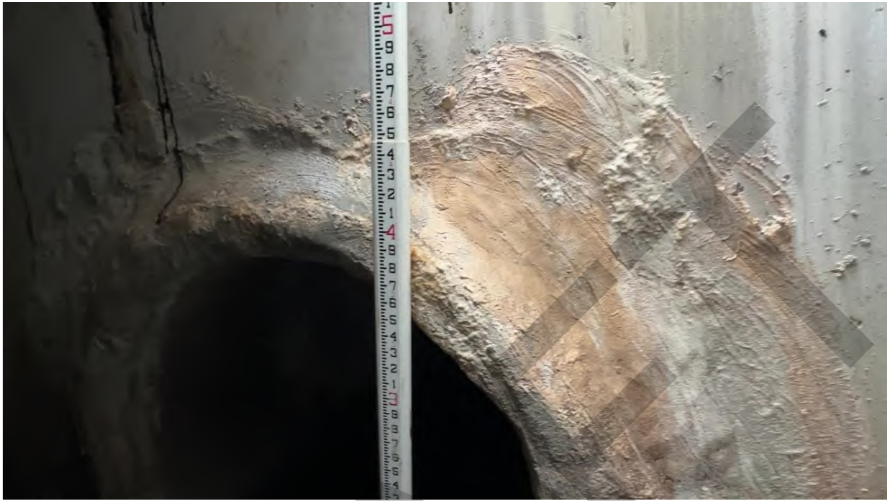
Intersection of W Morrison Ave and S Marti St where the 48"x76" ERCP constricts to a 48" RCP
